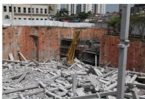
Advanced deterioration of structural components. The overhead slab is almost fully deteriorated with little remaining strength.
