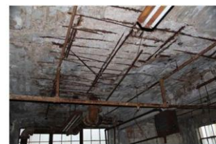
Building component failure. Image shows failing brick masonry arch, an imminent danger to the general public. Life safety is of paramount importance.
